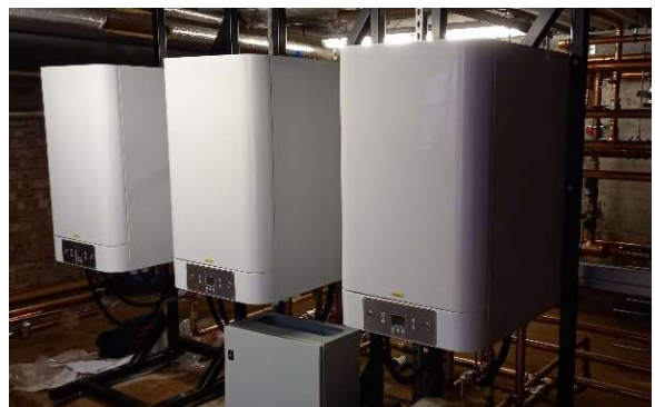
The new boilers in place
